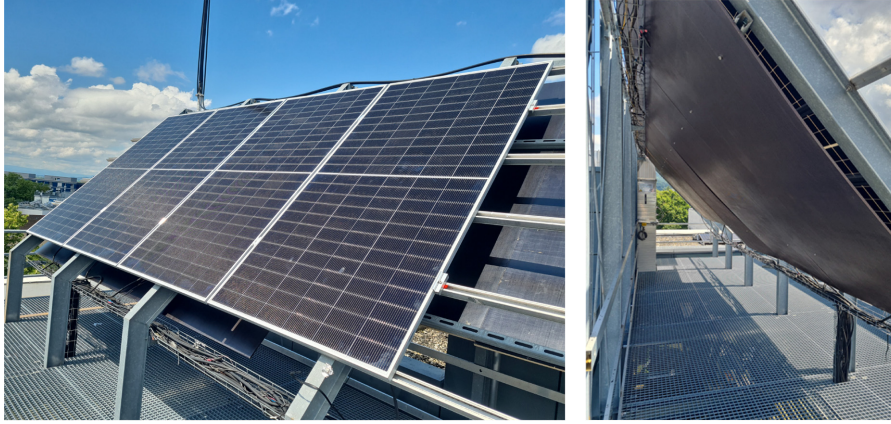
Fig. 1. Photographs of the outdoor installation on Site 1.
