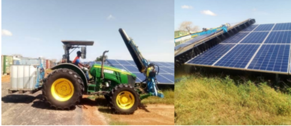
Fig. 1. Cleaning system of PV modules.
