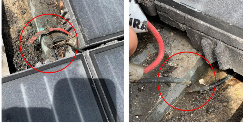
Fig. 6. Detected open-circuit positions at string 2.42 (left) and string 2.41 (right) with the signal transmission method.
